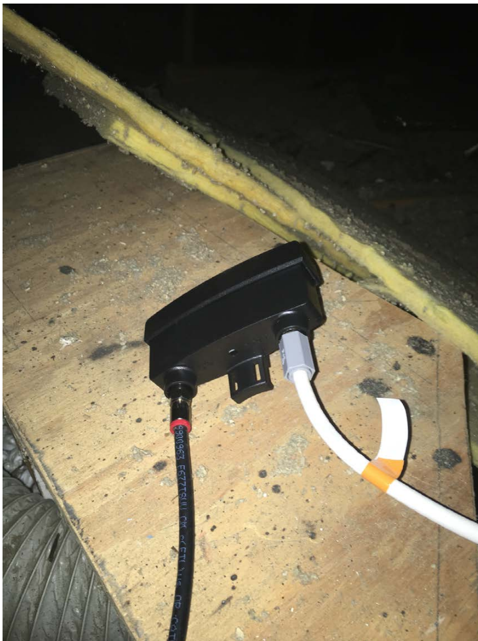
Figure 7. The preamp is as close to the antenna as possible.
