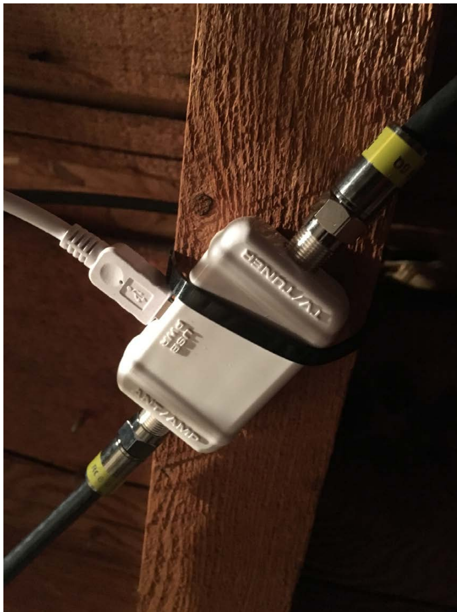
Figure 8. The power injector can be a bit away from the actual preamp.
